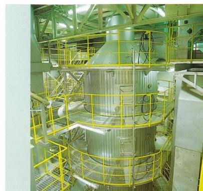
●減温塔 Cooling tower
